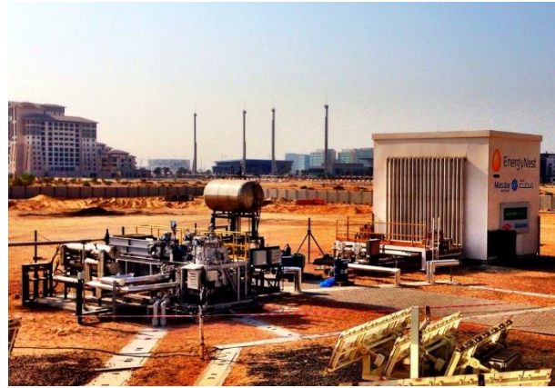
Fig. 2. Hot-oil loop (left) & EnergyNest TES pilot (right).
