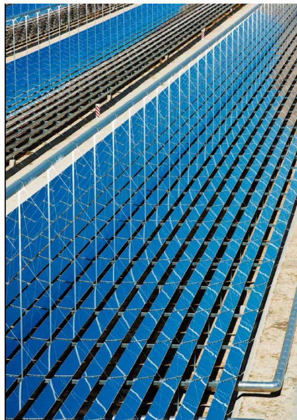
Figure 12: Novatec's Puerto Errado 2 (PE2), a 30 MW solar thermal power station in operation since August 2012 in Spain.
